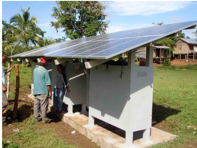
Fig. 1. One of the three PV battery charging stations (NW system) at Francia Sirpi.
