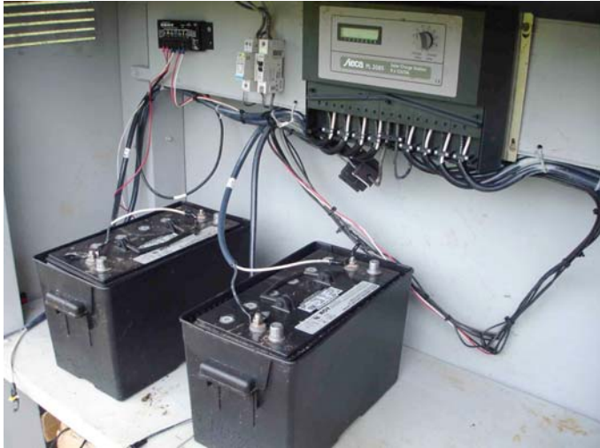
Fig. 2. Battery charging at Francia Sirpi with Stecca controller capable of charging 8 batteries simultaneously.
