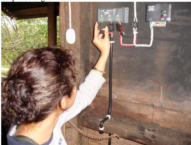
Fig. 3. CNE engineer inspecting the charge controller used as a LVD for a household lighting system in Francia Sirpi.
