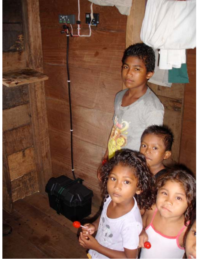
Fig. 4. Home kit with deep-cycle battery safeguarded in a battery box against the most curious PV system clients.
